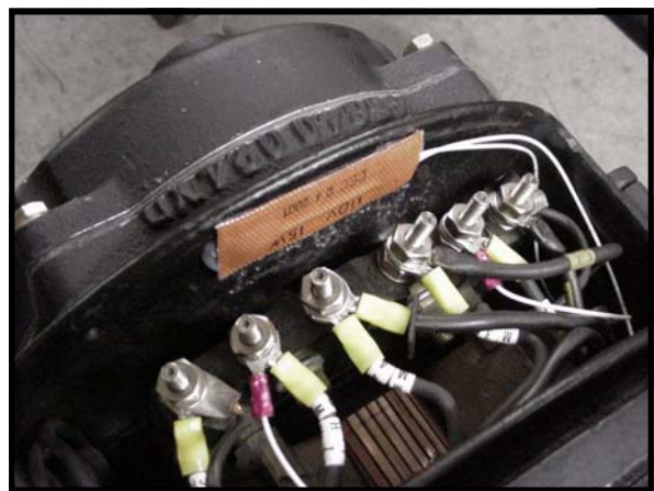
Typical Heater Installation in GRS Model 5 Switch Machine Motor
